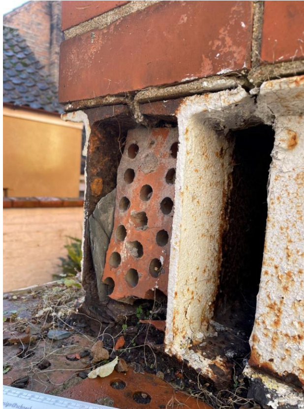
Figure 4: Heavy corrosion in outside steel above SE column
