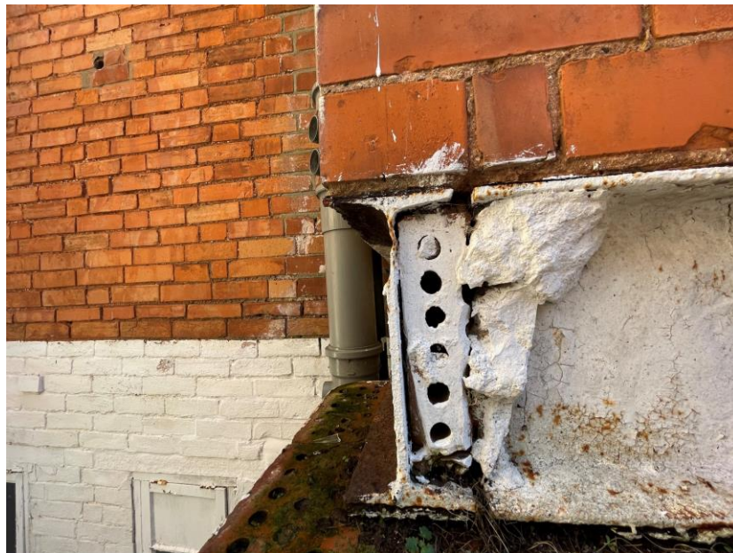
Figure 5: Web Buckling in steel above SW column (viewed from the south)
